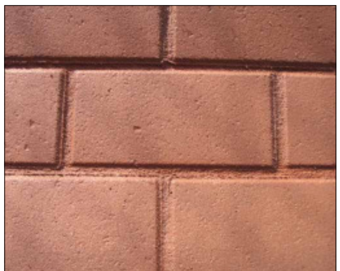
3 Exposed chamfer at joints, with colour of Sopro BSF 611 matching concrete pavers through addition of pigment.
