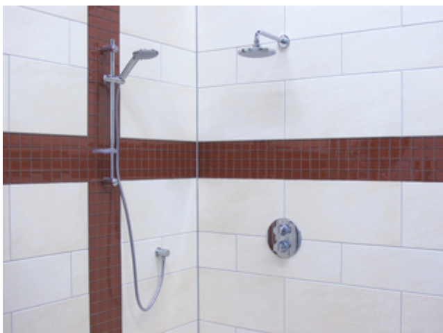
11 Brilliantly coloured joint surfaces in bathroom.
