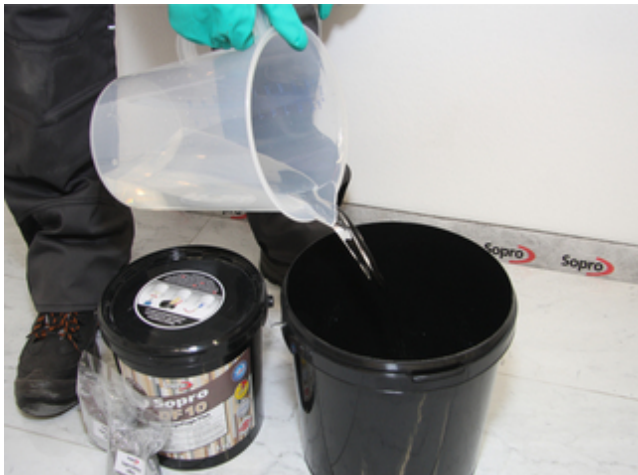
1 Fill clean bucket with clean mains water.
